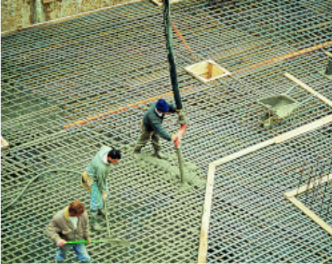
Detail of casting of foundation bed with superfluid concrete admixed with Mapefluid PZ500
